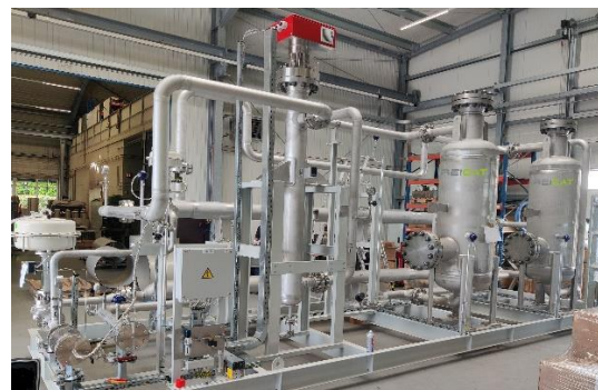
CO 2 Purification 3.000 Nm 3 /h
